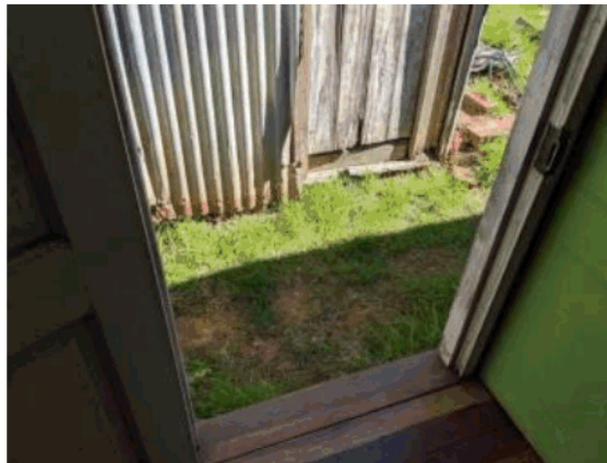
Plate 14: Separation between kitchen building and skillion
